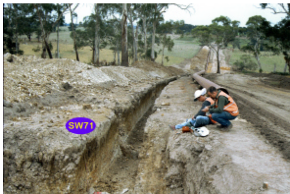
View from site SW71 westwards along pipeline easement (SW70 is on the distant slope).
